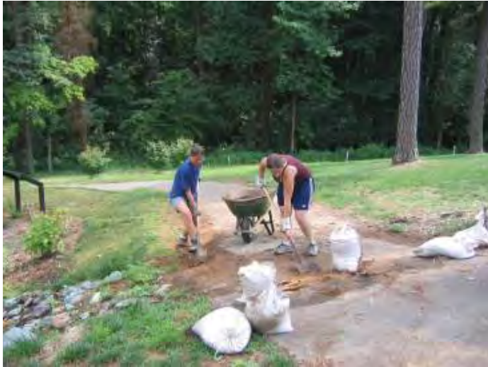
Remove sediment from inlets, curb cuts, pavement edges
