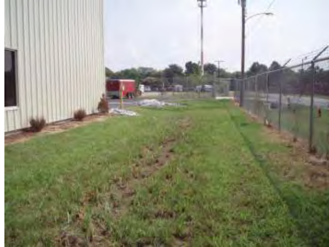
Sparse, ground too soggy
