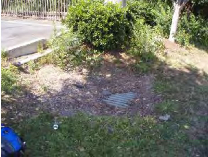
Debris from Curb Cut Blocks Outlet
