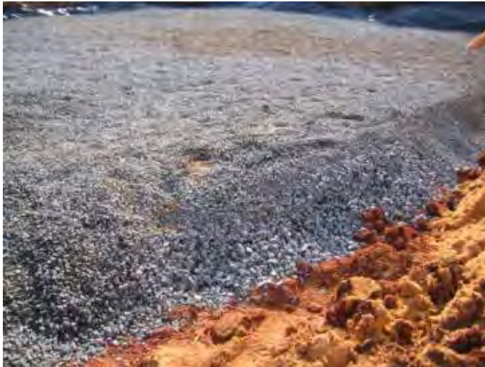
Add 3" choker stone (#8 or #89) on top of underdrain stone instead of filter fabric
