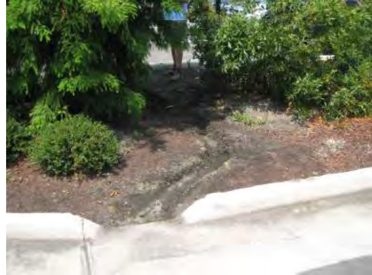
Flow from Curb Cut Creates By-Pass Channel
