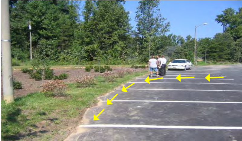
Sediment buildup at grass edge diverts flow
