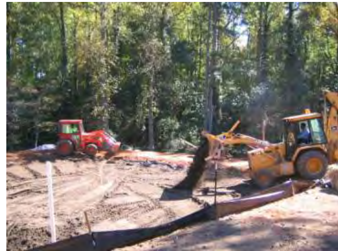
Add soil media in 12" lifts from sides. Bring to design elevation and add more after settling
