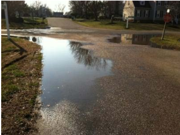
Figure 2.2a2b. Lack of Gravel Diaphragm
